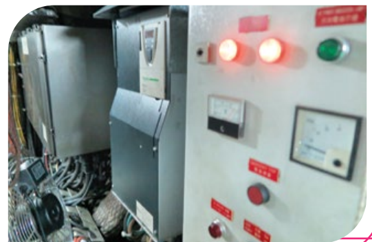
Installation of variable frequency inverters to enhance energy efficiency 安裝變頻器以提高能源效率
